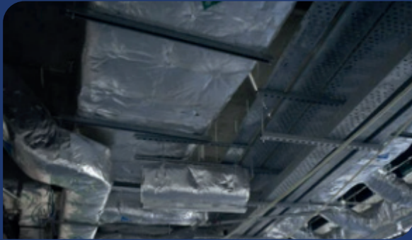
Mechanical, electrical and plumbing (MEP)
