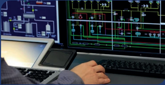
Building management system
